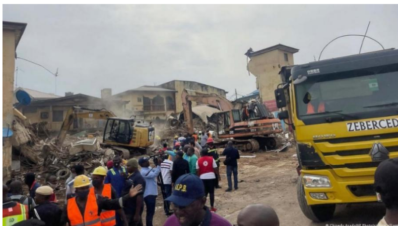
Plate 1: Two Storey Building Collapse in Garki Village, Abuja – 24 th August, 2023.
