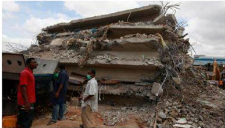
Plate 2: Multi-Storey Building Collapse in Gwarinpa, Abuja – 2 nd February, 2023.
