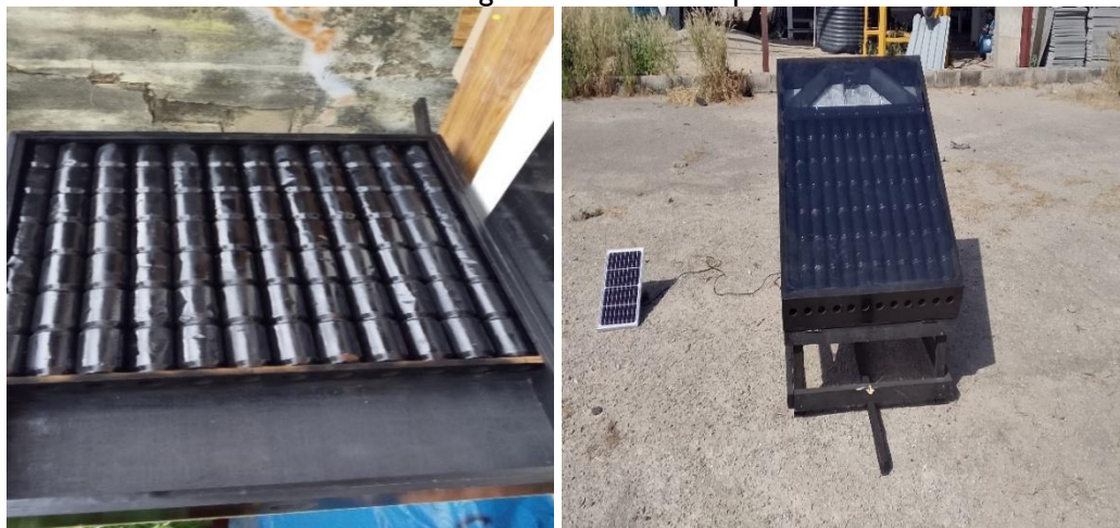
Plate 1: Collector absorber tube (cans) configurations (a), completed installation of all SAH components (b)
